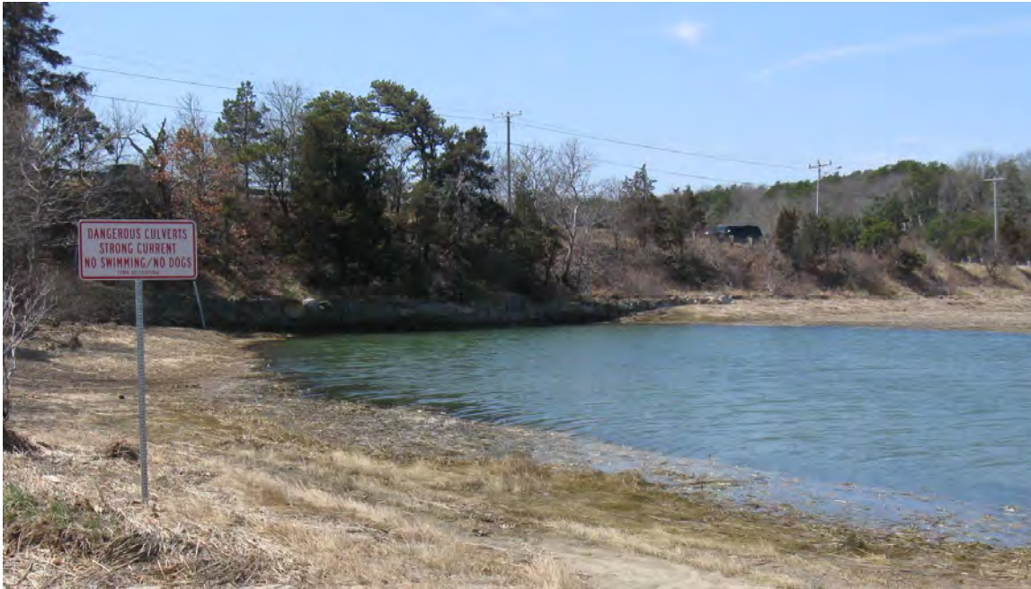
Figure 6 – Photo of Earthen Embankment and Culverts at Orleans Road/Route 28 Crossing over Muddy Creek Facing West Toward Harwich (April 15, 2011).
