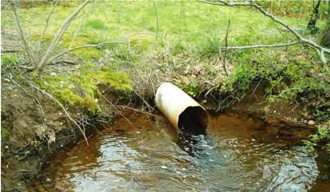
Figure 8 – Culvert Discharging Flow from Minister's Pond to Muddy Creek (18" CMP) with Eel Passage Ramp Substrate (submerged)
