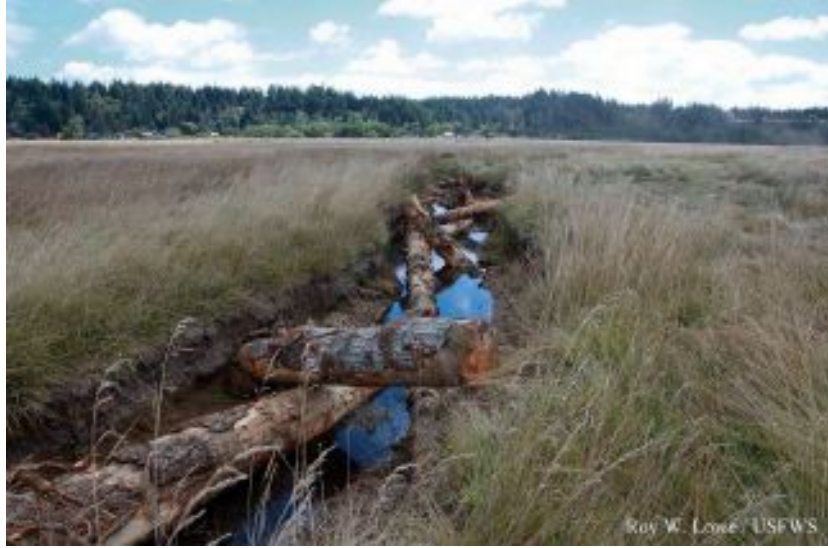
Figure 4.6 Bandon's Ni-les'tun Marsh restored 400 acres of diked and drained pasture into a vibrant tidal marsh. The project created over 5 miles of new tidal channels and doubled the acreage of tidal marsh habitat in the estuary ( Photo Credit: Roy Lowe, USFWS ).
