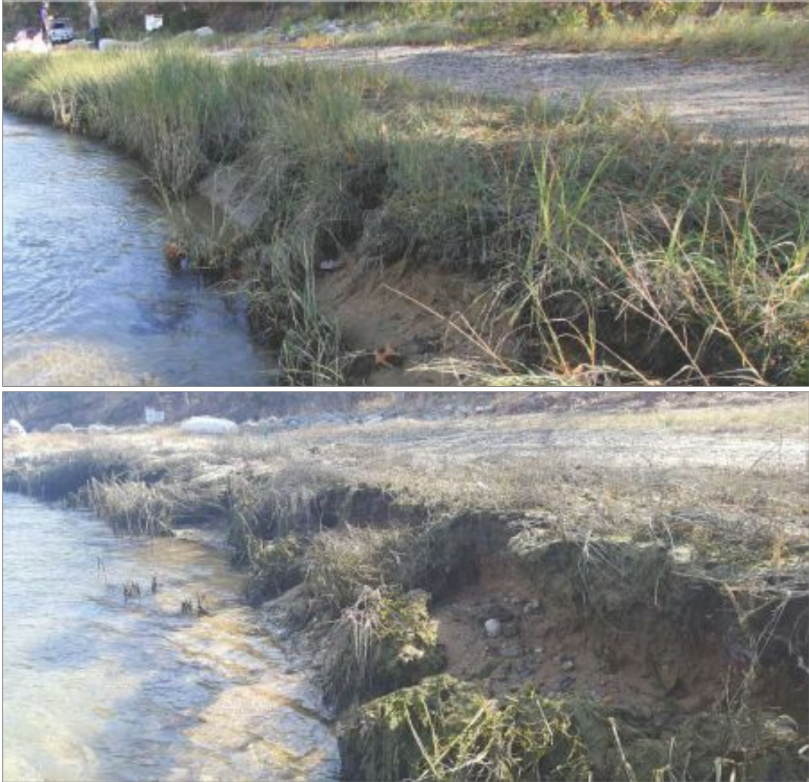
Figure 3.7 Photographs of the collapse of salt marsh bank between November 10, 2020 to March 31, 2021
