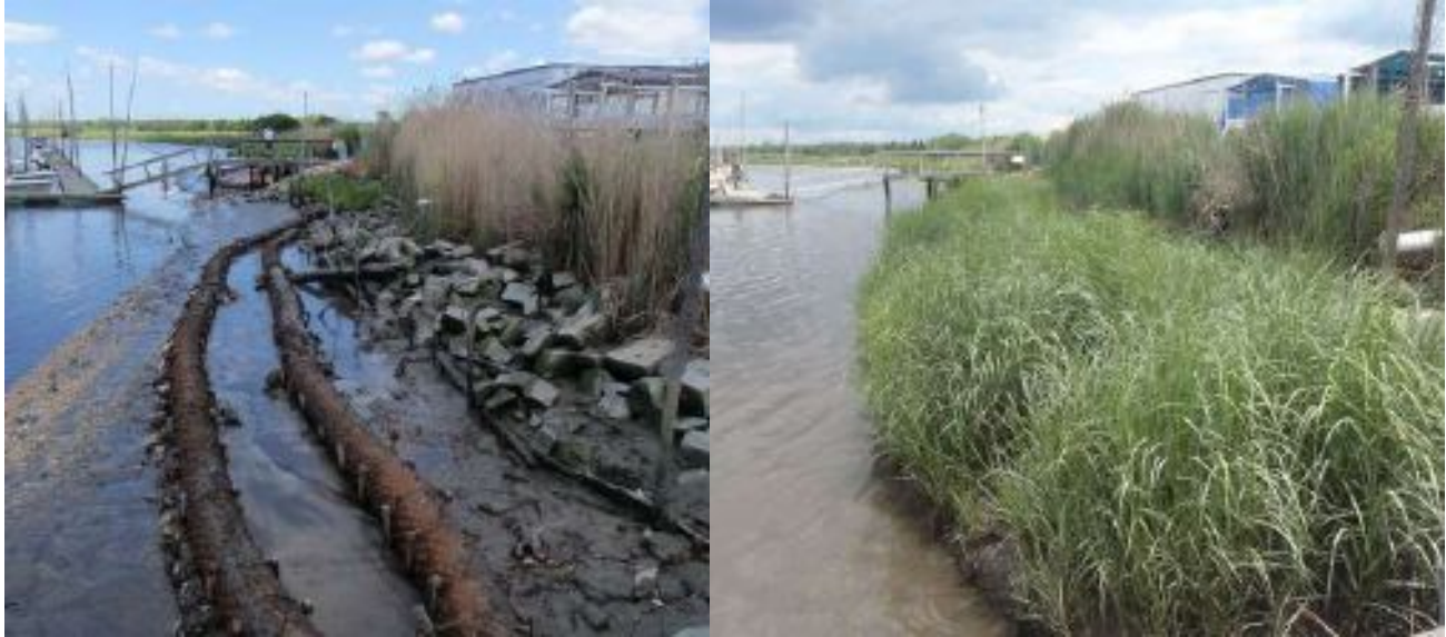
Figure 4.3 Installation of living shoreline in Delaware Bay with rock sill and core logs with the addition of oyster shells along seaward edge. Restoration site 1-Year after installation. (Photo Credit: Delaware Department of Natural Resources)
